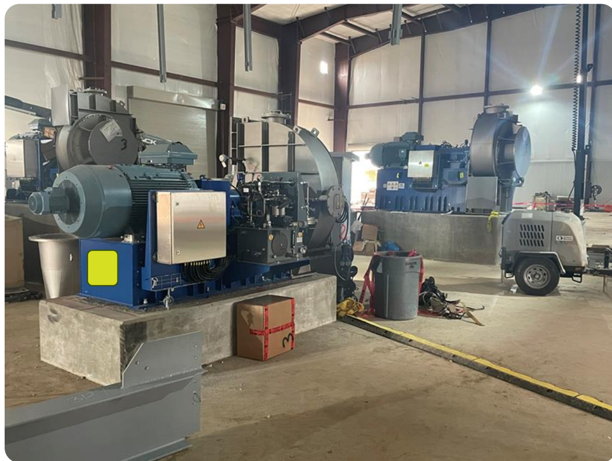
Permeate Vacuum Fans
